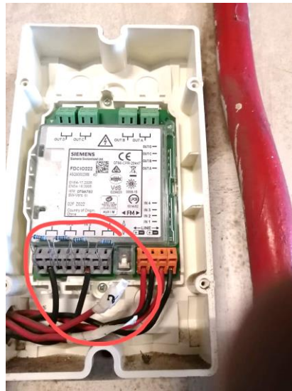
Picture A – Disconnected Link.
