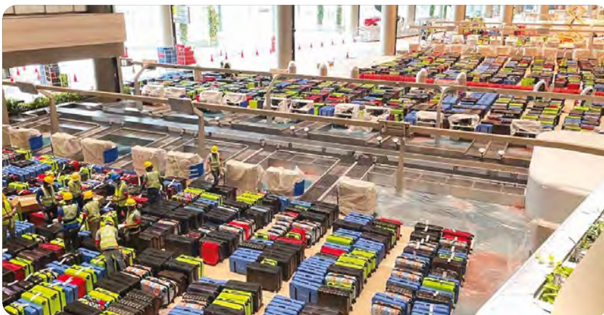
CAG conducted intensive tests of the upgraded baggage handling system at T2 before its reopening.
