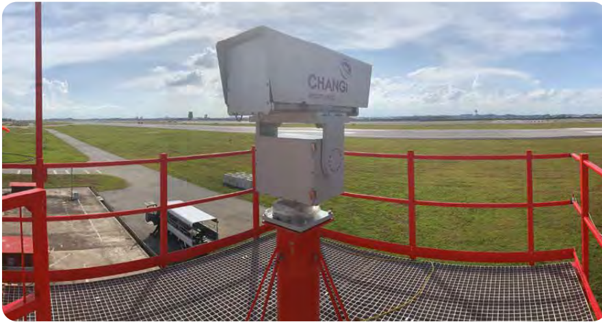
iFerret provides automated round-the-clock surveillance of the runway to reduce the threat of foreign object debris.
